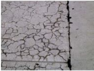
Damage of Asphalt
