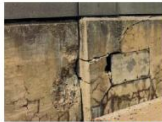
Damage of Wall Deck
